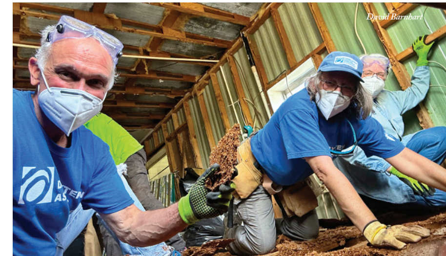
Jim Kirk, Kathy Broyard and Marilyn Stone remove flooring from a home impacted by Hurricane Ian.
