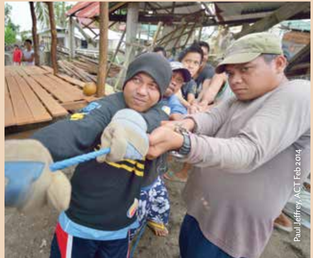
Men pull on a rope to guide a coconut tree that is being felled. The felled tree will be cut into lumber for the construction of temporary houses.
