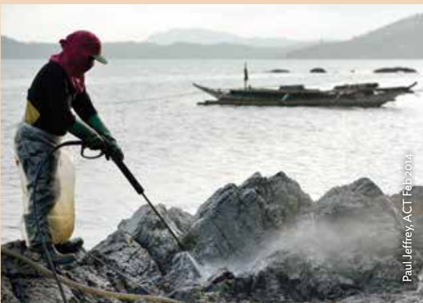
A worker sprays rocks along the shoreline in Botongon, a neighborhood of Estancia, Philippines, in an effort to remove oil that spilled there when Typhoon Haiyan swept through the area in November 2013. Most residents who lived along the affected coastline remain in temporary shelters, despite government efforts to get many to return.
